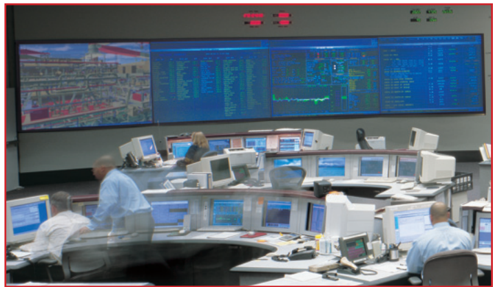
Figure 4. A collaborative work session using a 3D virtual model in the control room. (Courtesy of Newport Shipbuilding Inc.)
